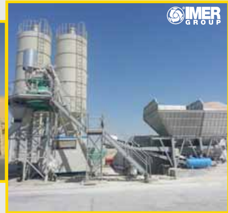
Concrete Batching Plants for Precast
