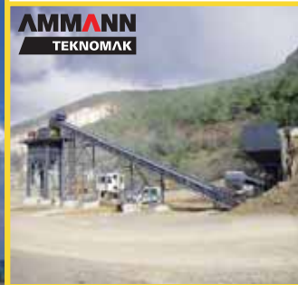
Base Stabilization Plants
